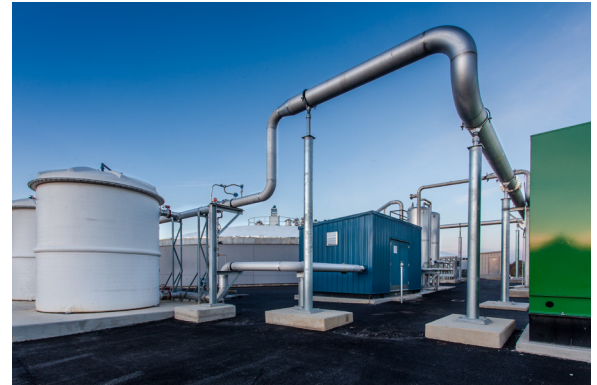
Above: Piping at the FWSA's Opequon facility that delivers biogas generated through anaerobic digestion to the facility's cogeneration system to generate electricity.
