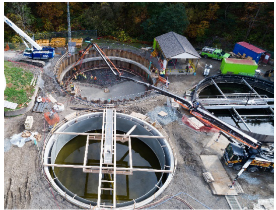
Above: ESG constructed two new secondary clarifiers at the Town of Niskayuna's wastewater treatment plant in addition to carrying out other major improvements.
