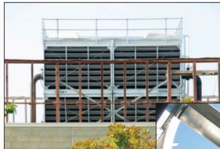
New Cooling Tower on Chiller Plant Roof
