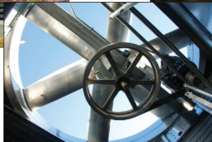
Fan Motor and Fan from Inside New Cooling Tower
