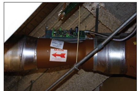
Phoenix Air Valve in overhead of BSB lab room
